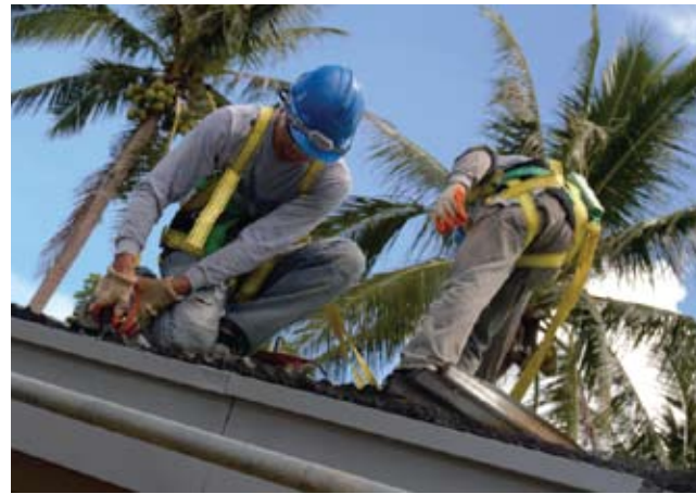
A PROJECT TEAM MEMBER AND A VOLUNTEER FROM THE PARENT-TEACHER ASSOCIATION WORK TOGETHER TO CLEAN THE SCHOOL'S ROOF GUTTERS
